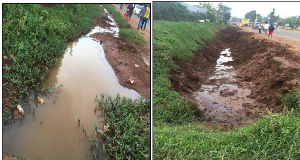
Figure 6: Ponding in Mwembe as a result of adverse slope
